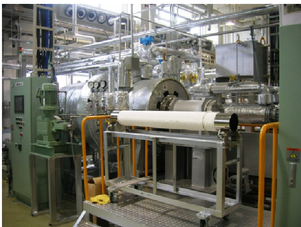
Fig.12 Practical supercritical fluid plant having 350 liter treating bath for fiber and textile treatments.
